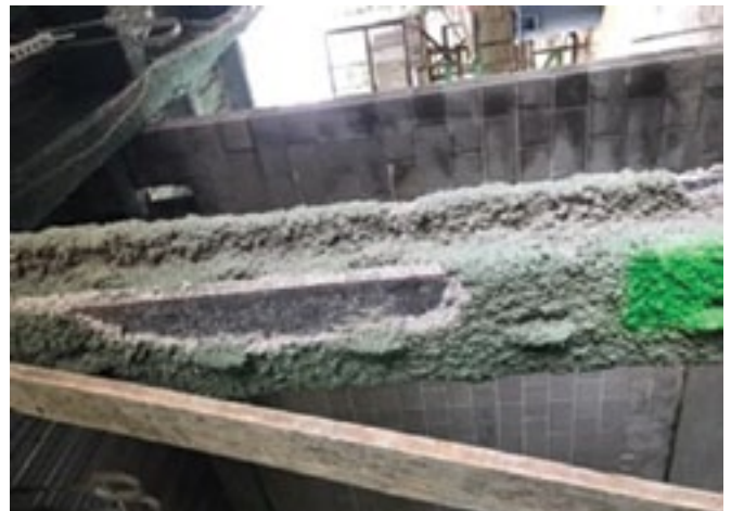
SFRM or IFRM can be damaged during construction, then repairs are needed. GCP Applied Technologies Photo
