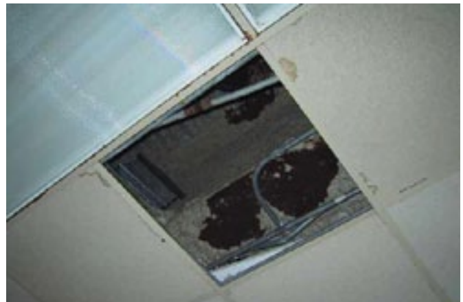
SFRM or IFRM can be damaged when new services are added to existing buildings and need repair and documentation of the repair to comply. GCP Applied Technologies Photo
